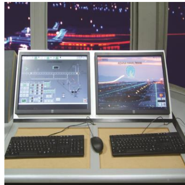
ALCMS Airport Lighting Control and Monitoring System
